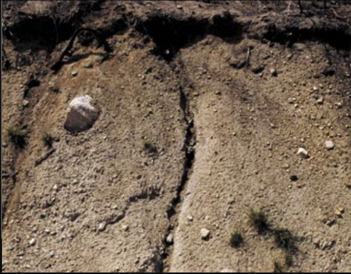
Erosion – Surface erosion.
