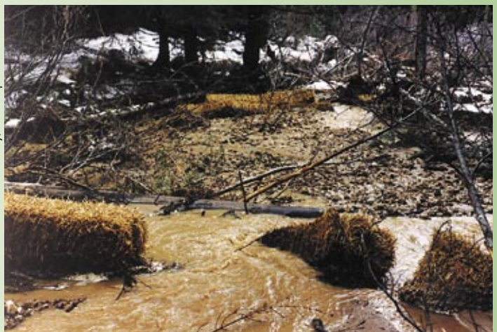
Failed straw bale check dam.
