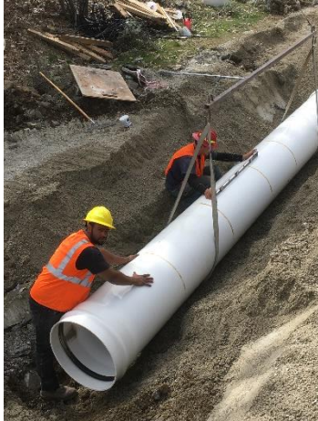
Open canal to pipeline conversion for a multi-user irrigation association servicing orchard and hay/pasture crops
